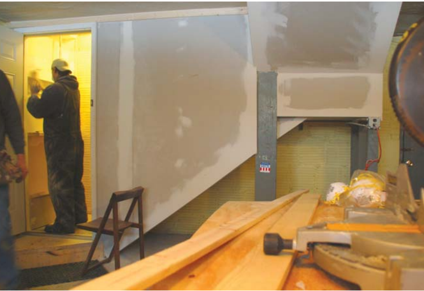
Jason Whitmarsh puts the final touches on a recently enclosed stairway, once a massive chase between unconditioned and conditioned space.
