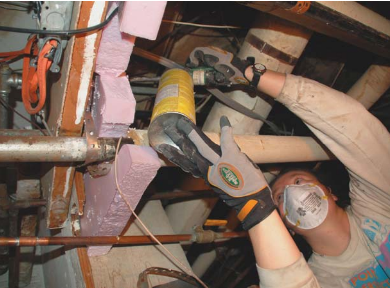
Lexie Hain works to create an airtight closure for an above-grade crawlspace.
